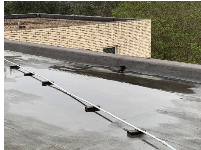
Water ponding on roof near drain
