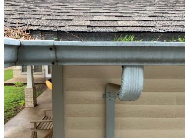
Vegetation in gutter
