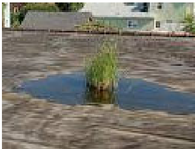
Vegetation around scupper
