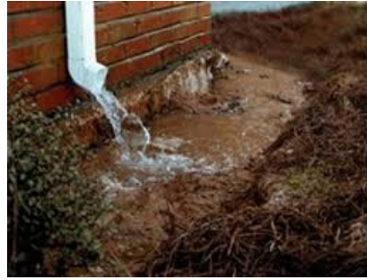
Water not being drawn away from building
