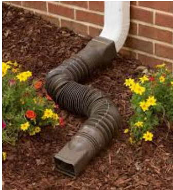
Downspout extensions can help move water further away from the building.
