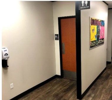
Wall blocking view of women's restroom door entrance
